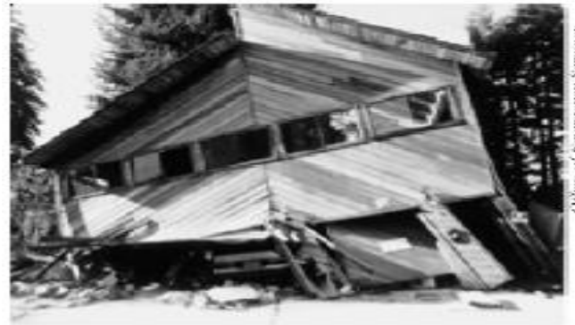
Figure 29 - This mountain home was built over a garage, and its walls were not strong enough to withstand an earthquake.
