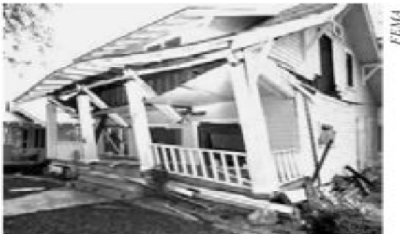
Figure 3 - Northridge Earthquake, Jan. 17, 1994 Single family residence damaged due to failure of multiple elements.
