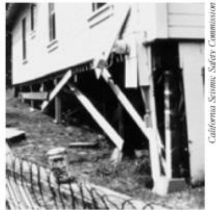
Figure 18 - The pier-and-post foundation under this home shifted during a recent earthquake.
