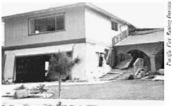
Figure 1 - San Fernando Earthquake, Feb. 9, 1971 Severely damaged split level 1 and 2 story wood frame dwelling. The one story portion dropped about 3 feet.
