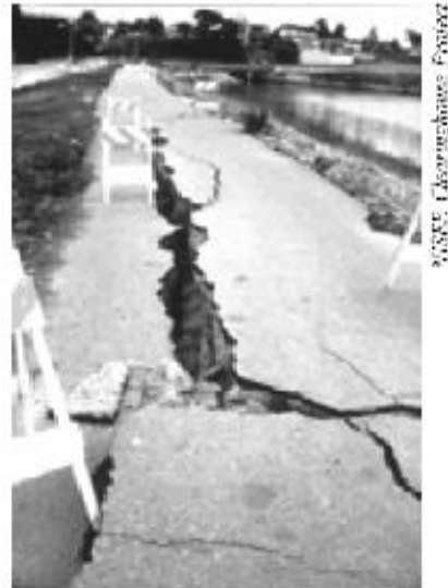
Figure 39 - Lateral Spreading. Loma Prieta Earthquake, October 17, 1989. Lateral spreading damage levee road along the San Lorenzo River.
