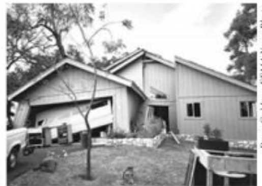
Figure 5 - San Simeon Earthquake, Dec. 22, 2003 This home slid two feet off its foundation due to inadequate nailing of walls to its sill plates.
