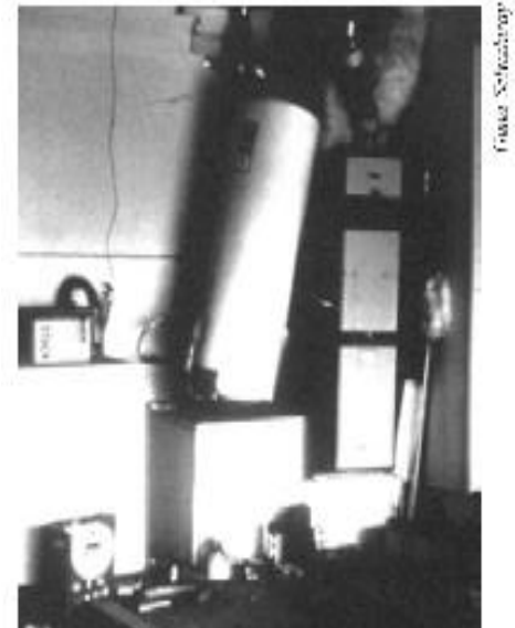
Figure 11 - This unstrapped water heater tipped over during the 1984 Morgan Hill Earthquake. Fortunately gas and water lines were not ruptured
