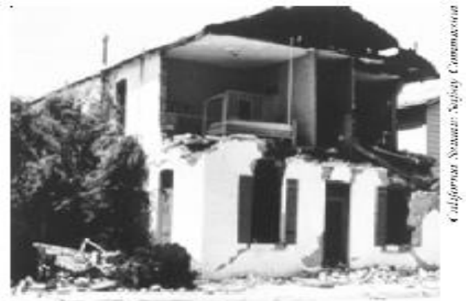
Figure 25 - The plaster-covered brick walls of this building collapsed during a recent earthquake.
