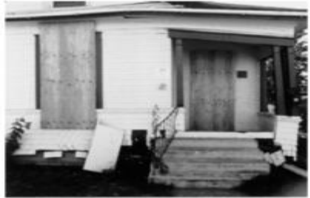
Figure 13 - This home wasn't bolted and slid off its foundation. Sometimes the damage can be so bad that houses have to be demolished.
