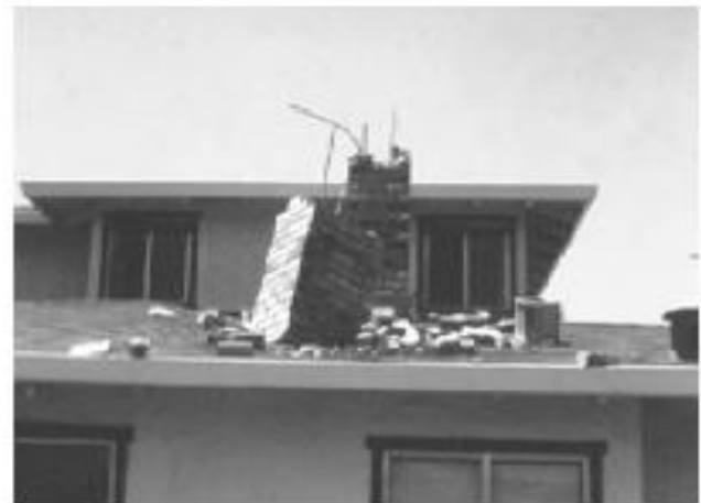
Figure 34 - Morgan Hill Earthquake. Broken chimney fell on roof.
